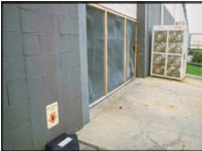
Figure 3. Food safety demands a partnership between pest professionals and food clients. This exterior bait station, no matter how well placed and well baited, will not prevent rodents from freely entering into the distribution center through this decrepit screen door. Should that happen, the pest professional is often held “to task” for getting rid of the interior infestation of mice that has developed.
